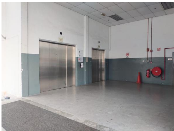
Loading Bay and Cargo lift
